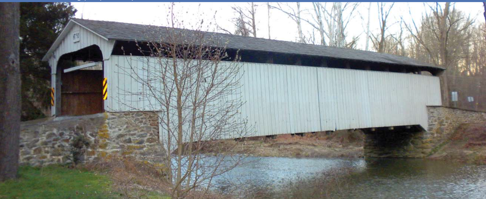
The Rudolph and Arthur Covered Bridge in New London and Elk townships, respectively, was selected for the FY 2009 National Historic Covered Bridge Preservation Program .
